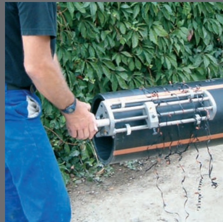
Optimum removal of the oxidic layer: a FRIATOOLS scraper tool being used.
